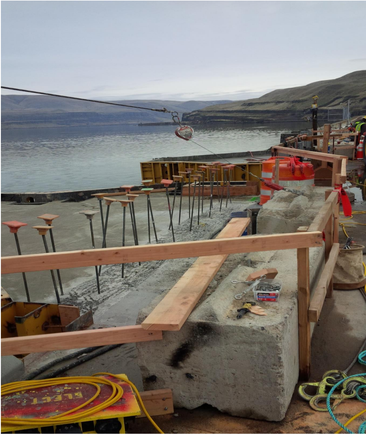
Capping the AWS intake slot
